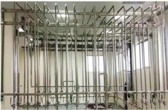
Process Piping - Food Industry
